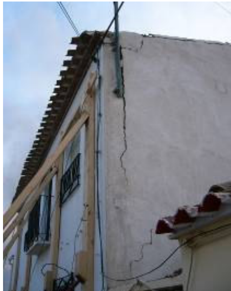
Drift of walls in blockwork construction. Zarcilla (Grade 2 vulnerability B)
