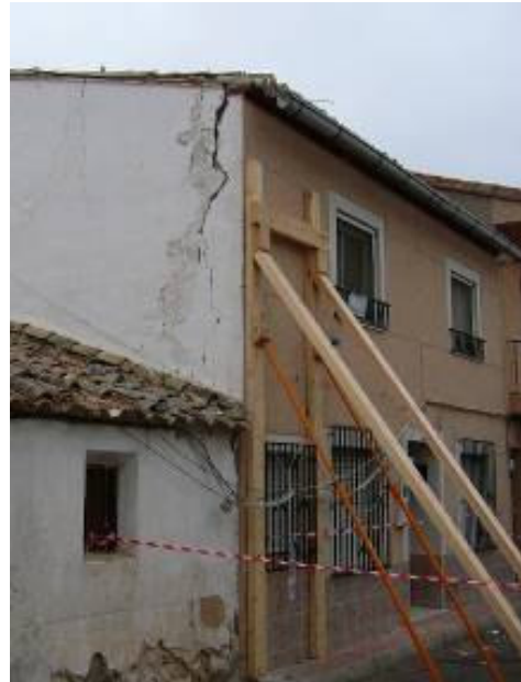
Drift of load bearing masonry in composite construction. La Paca. Note repairs from the 2002 earthquake (Grade 2vulnerability B)
