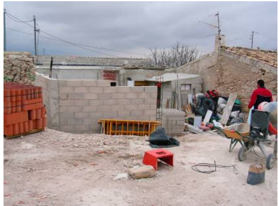
Hours after the earthquake a homeowner embarks in self-reconstruction using sub standard materials and poor technical knowledge. There is probably no planning permission for this hazardous job which will be surely damaged in the future.
