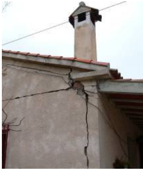
Heavy Drift of many elements in blockwork construction. La Paca (Grade 3 vulnerability B)
