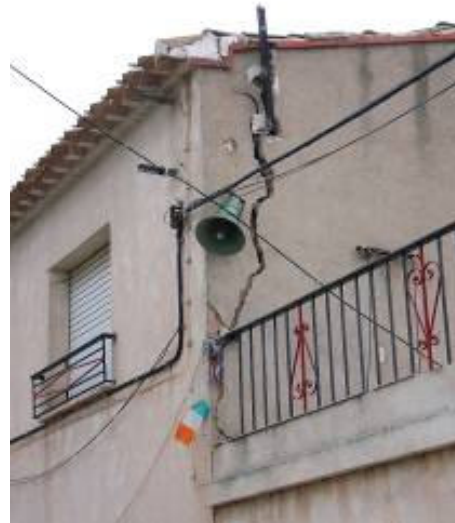
Heavy Drift of walls in blockwork construction. La paca (Grade 3vulnerability B)
