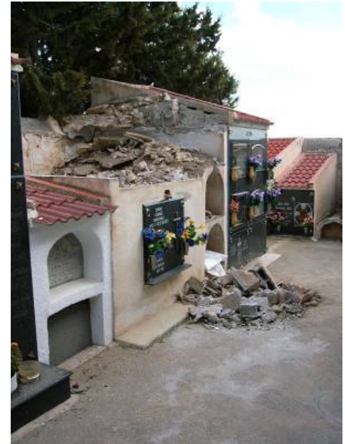
Damage to niche structures in Zarcilla
