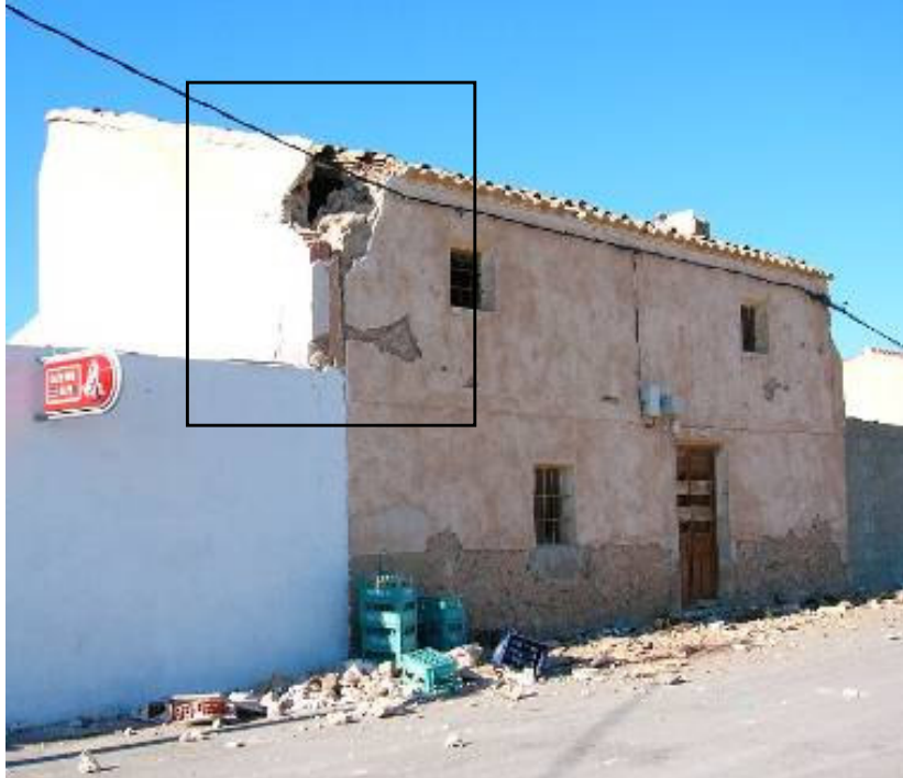
Corner failure in masonry construction in Zarçilla. (Grade 3 vulnerability B)
