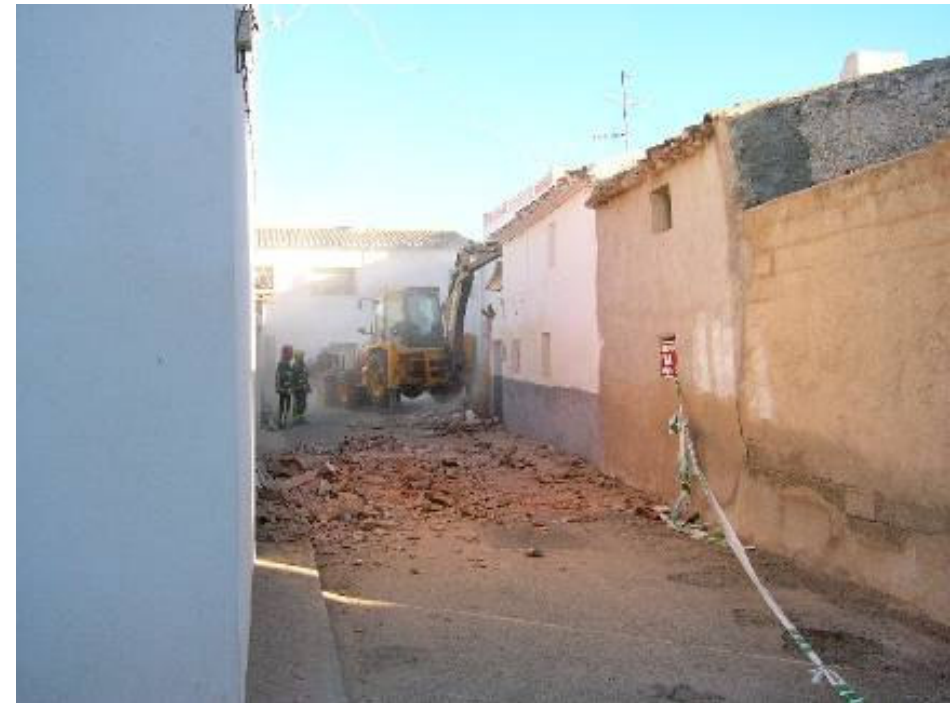
Removing rubble the day after the earthquake. Zarcilla
