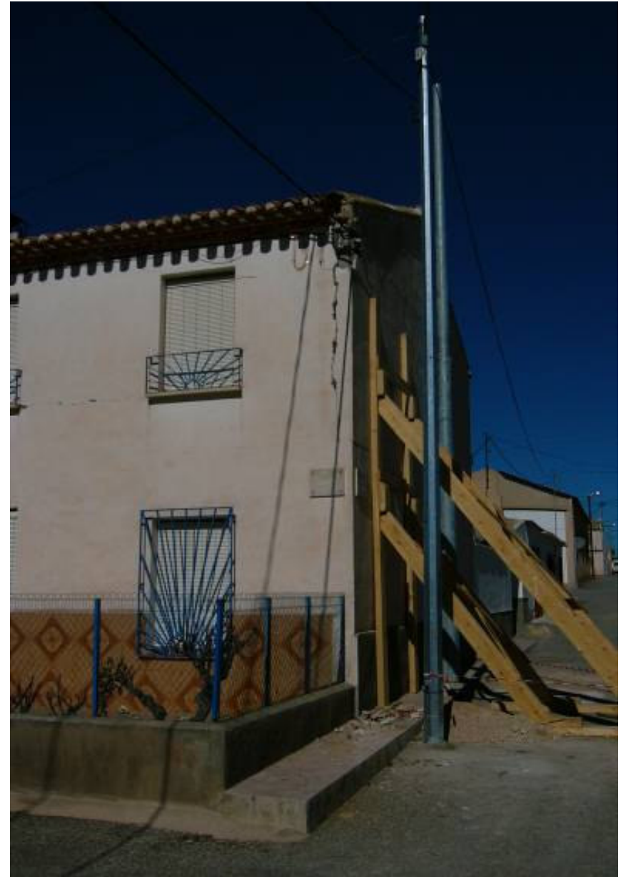
Drift of walls in blockwork construction. Zarcilla (Grade 2vulnerability B)
