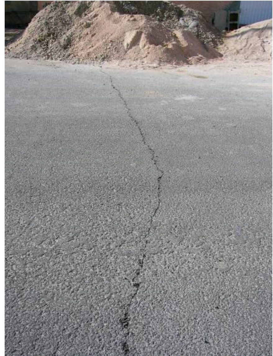
Cracking in streets of La Paca (left) and Zarcilla (right)
