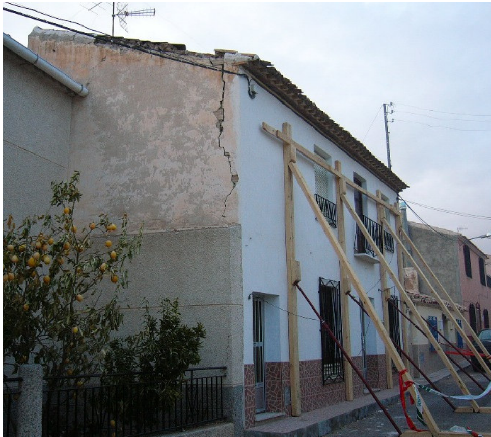
Drift of load bearing masonry in Zarcilla. (Grade 2 vulnerability B)
