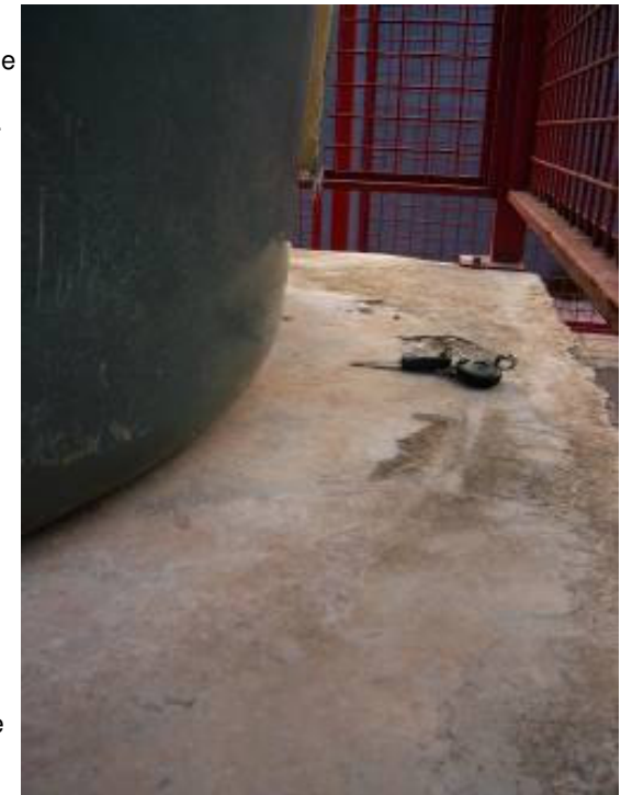
Marks on the concrete pedestal leave a tell-tale story of the tank's displacement
