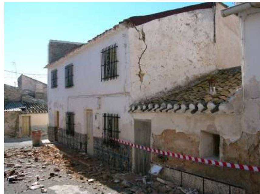
Drift of load bearing masonry façade. Zarcilla (Grade 2 vulnerability A)
