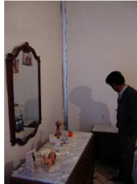
Drift of bearing walls also affects internal partitioning as in this building in Zarcilla. (Grade 2 vulnerability B)
