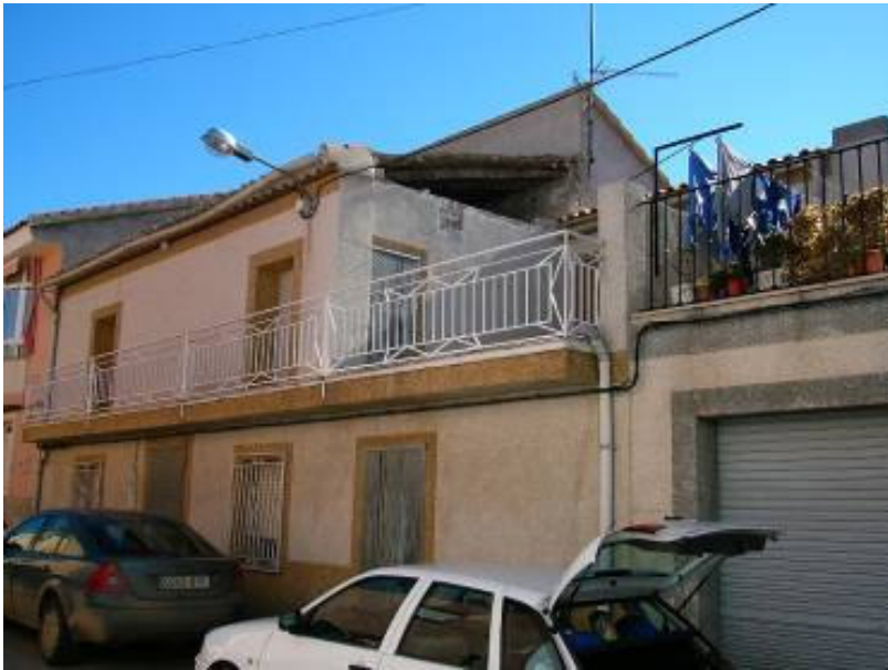
Gable wall failures from various homes in La Paca and Zarcilla (Grade 3 vulnerability As and Bs)
