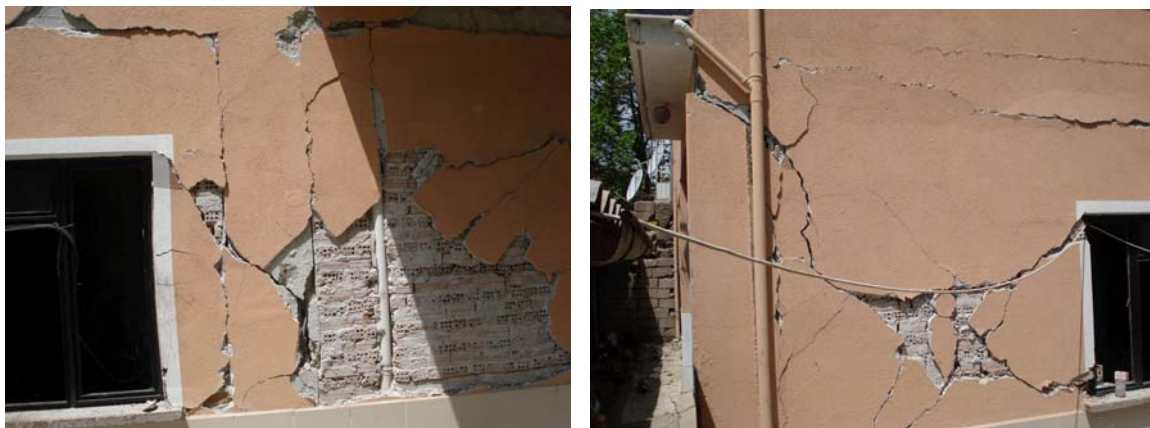
Figure 53: Same building with previous picture, similar damage pattern
