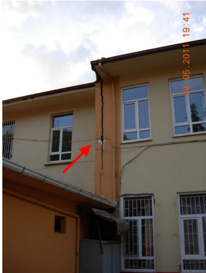
Figure 79: Large crack between masonry and RC parts of the school building
