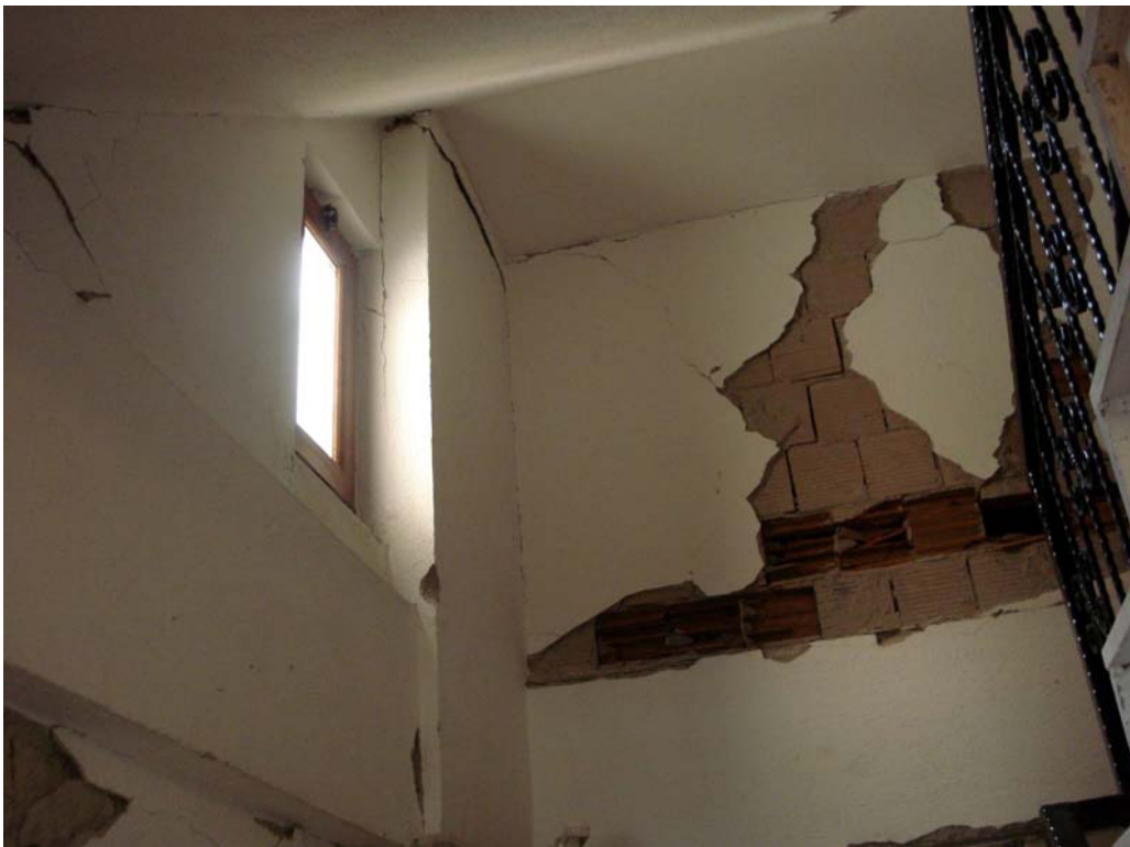
Figure 72: Building next to hospital complex – staircase infill wall cracks, spalling of plaster
