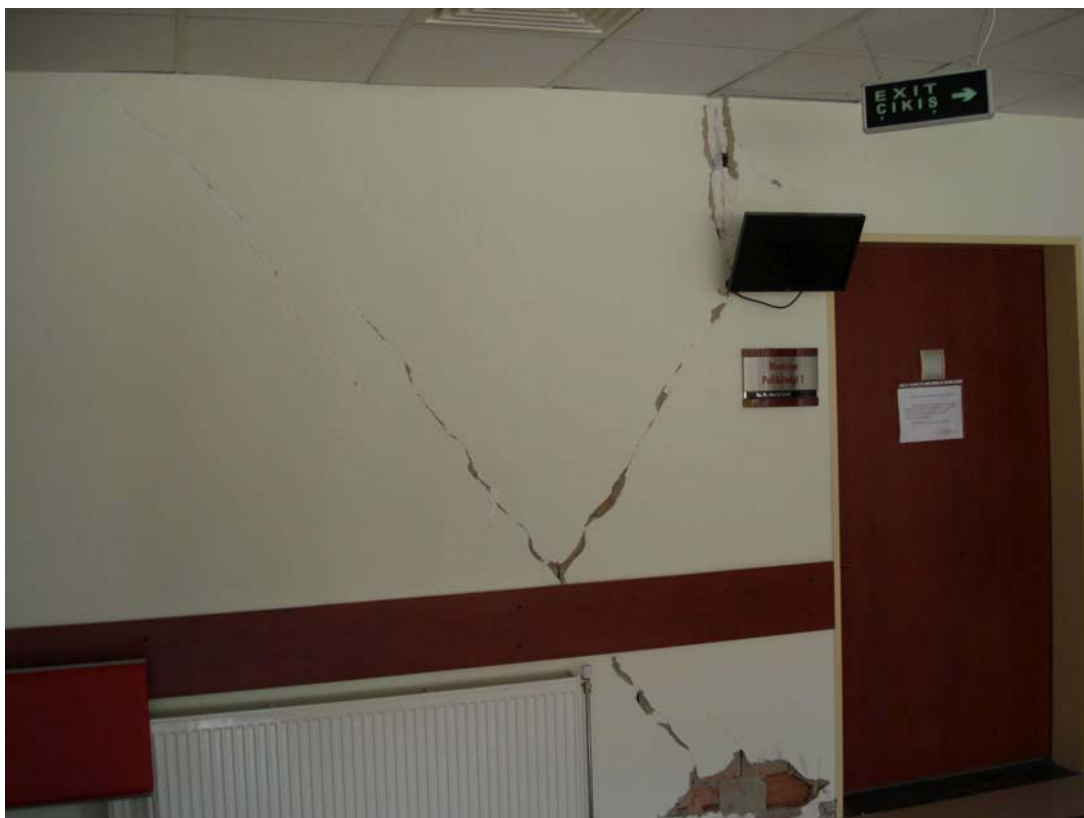
Figure 66: Recently completed building of hospital complex, cracks at infill walls, but building is still at operational level
