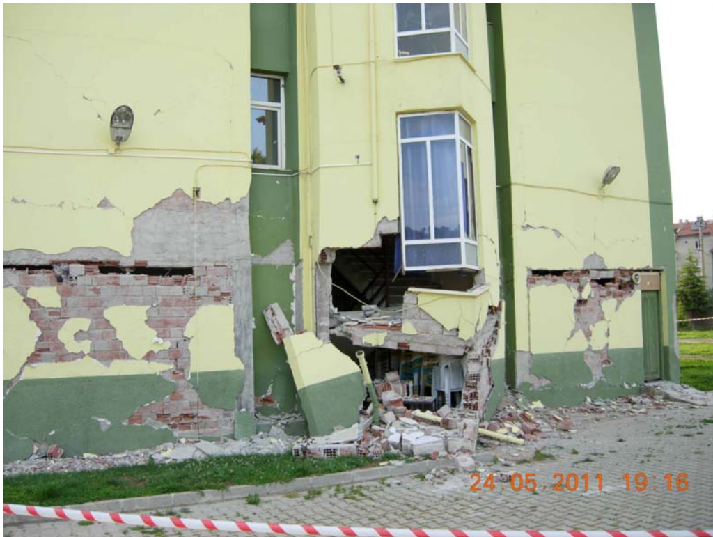
Figure 75: Staircase damage of the RC part of school building, general practice of the territory is to build staircase slabs so thin and without any beam to support the slab
