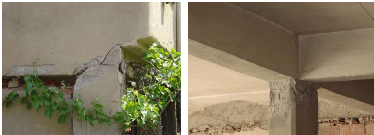
Figure 54: Heavy structural damage at column ends
