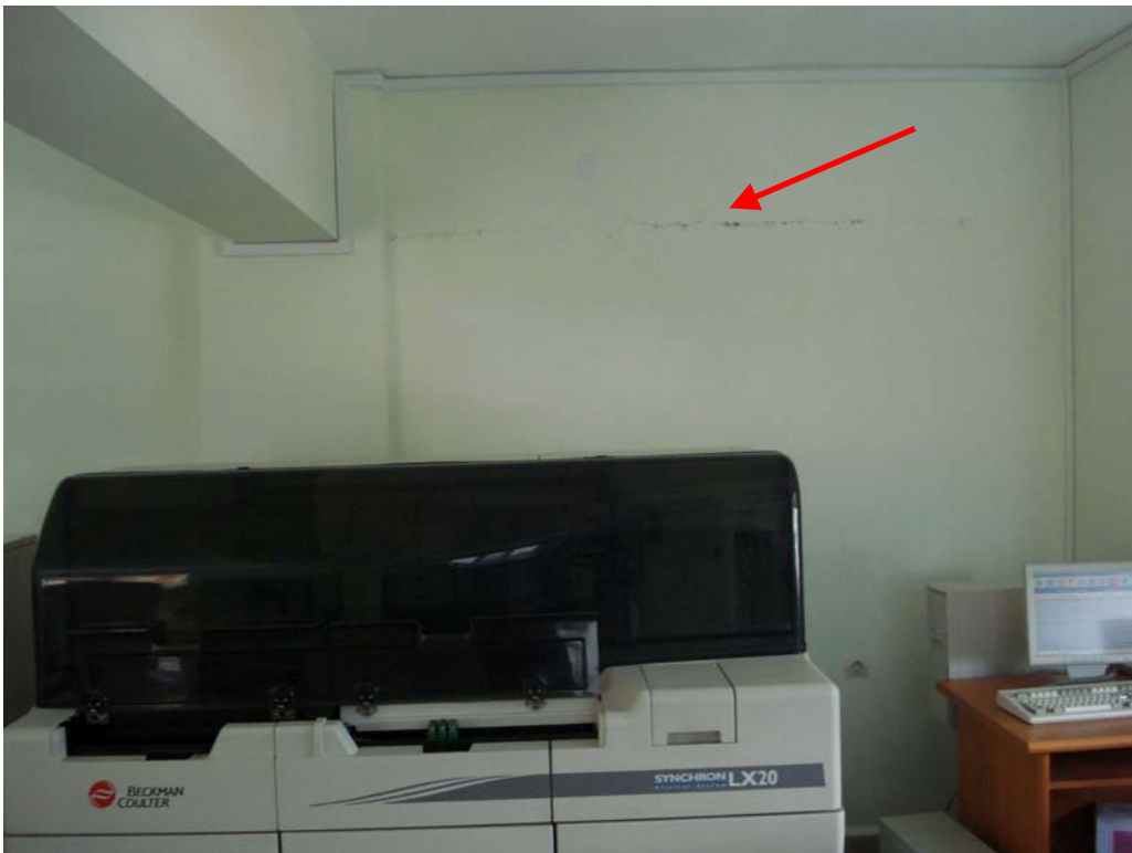
Figure 68: Hospital building, completed in the beginning of 2000's, biochemistry lab. (same room) , machine has displaced, and infill wall cracked during earthquake
