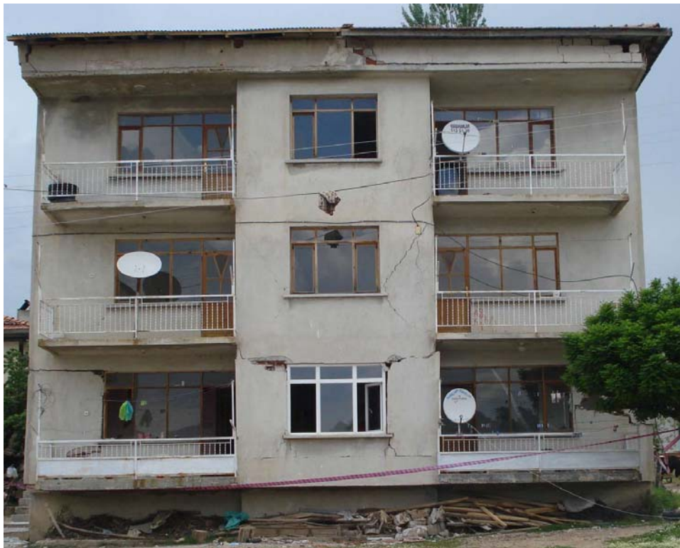
Figure 80: Gökçeler village, grade 3 damaged building, front view
