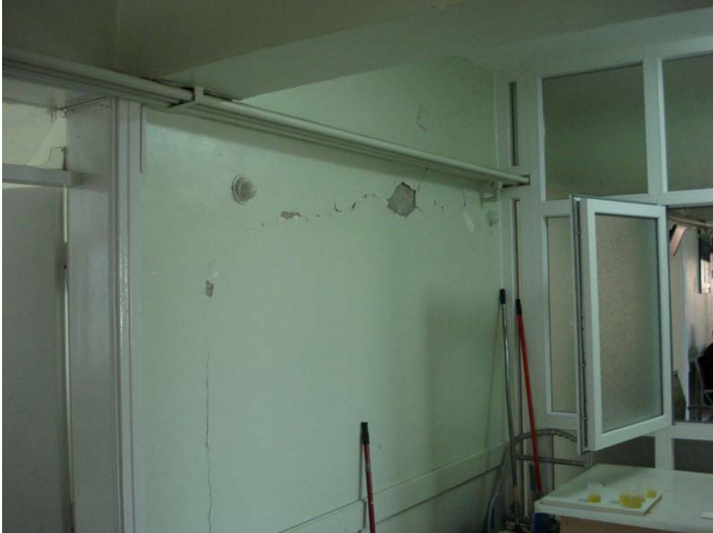
Figure 71: Hospital building, completed in the beginning of 2000's, infill wall crack
