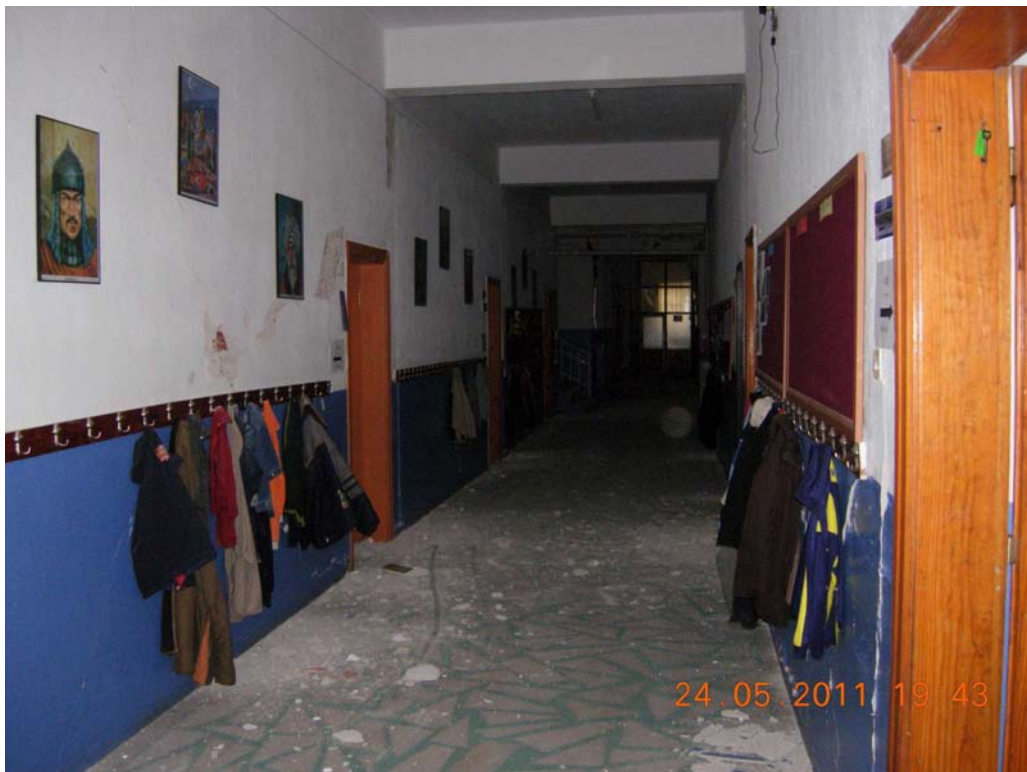
Figure 78: Inside of masonry part of the school building- spalling of plaster
