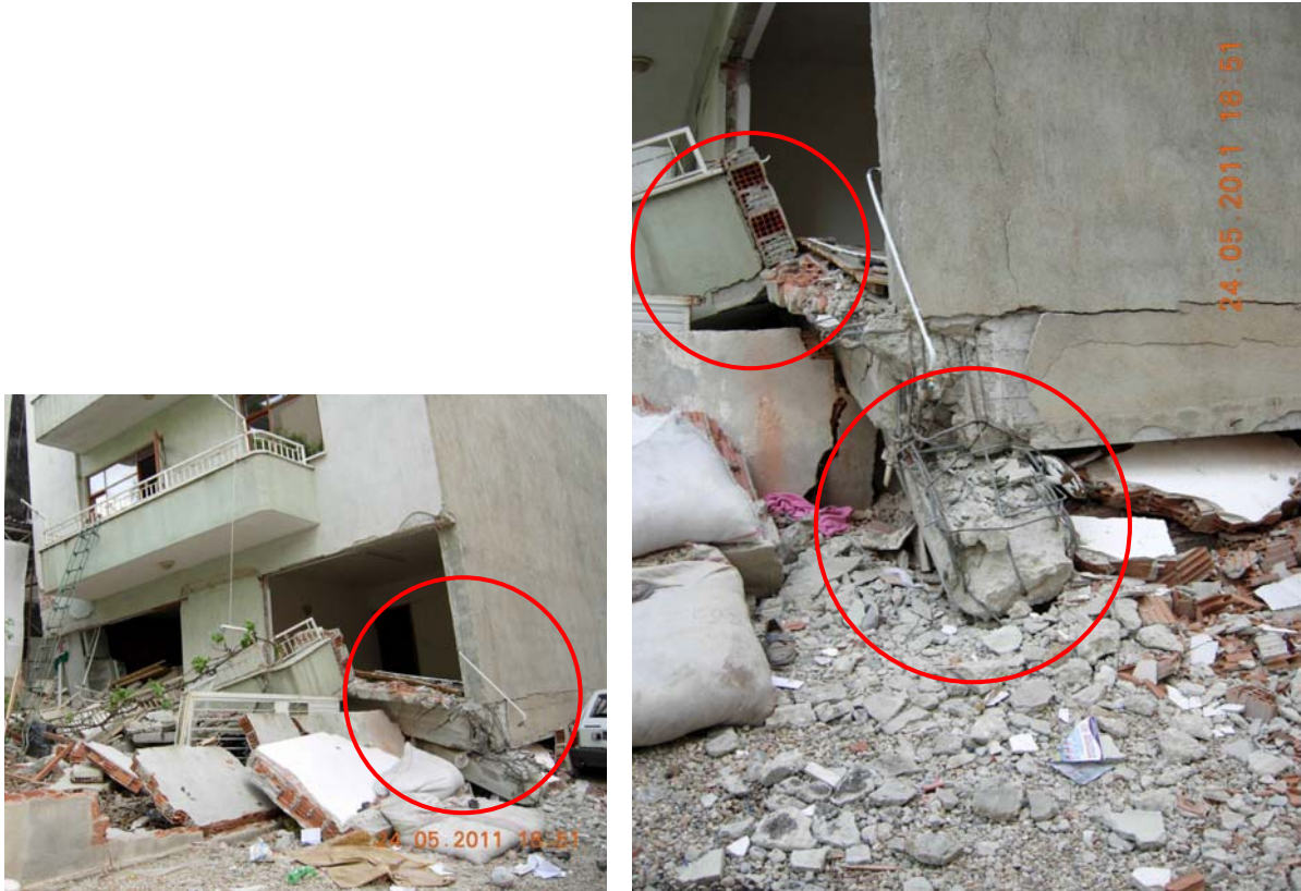
Figure 50: North-west corner column of the collapsed building
