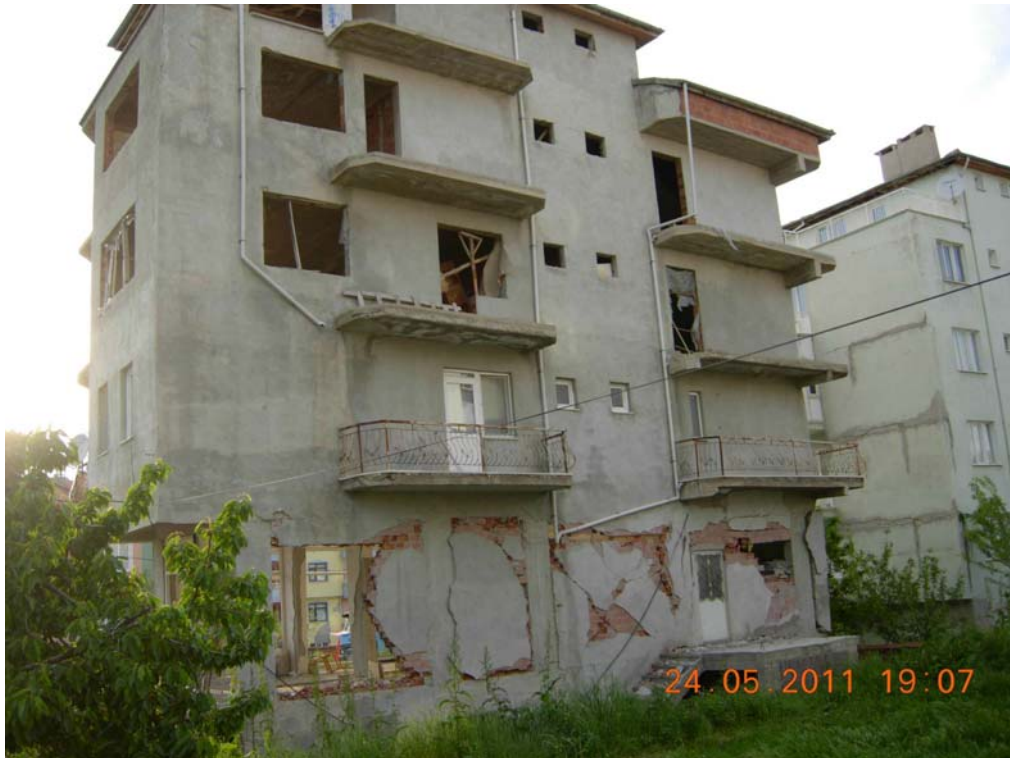
Figure 58: Non-structural infill wall damage on a new building which is still under construction
