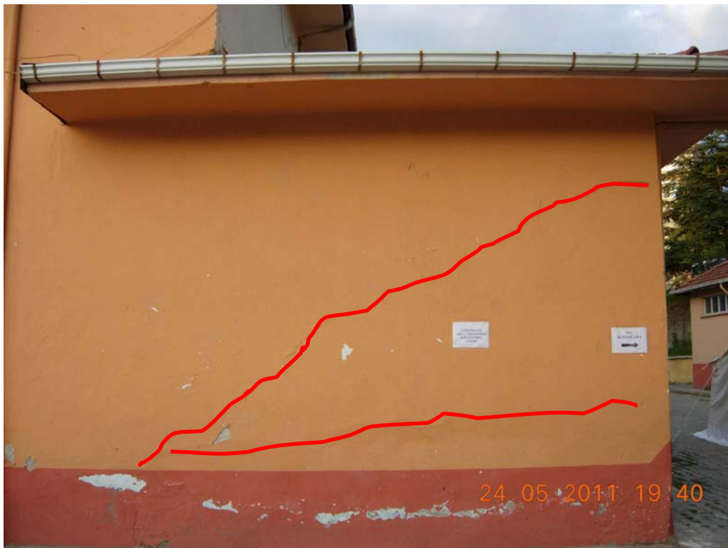
Figure 76: Cracks on outer walls of masonry part of the school building
