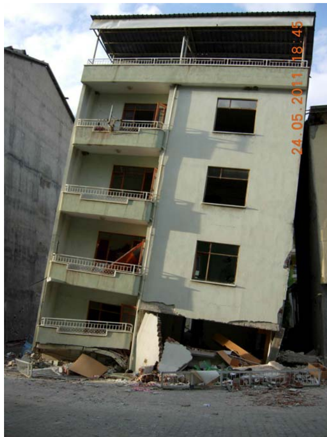
Figure 47: Collapsed building at the town center
