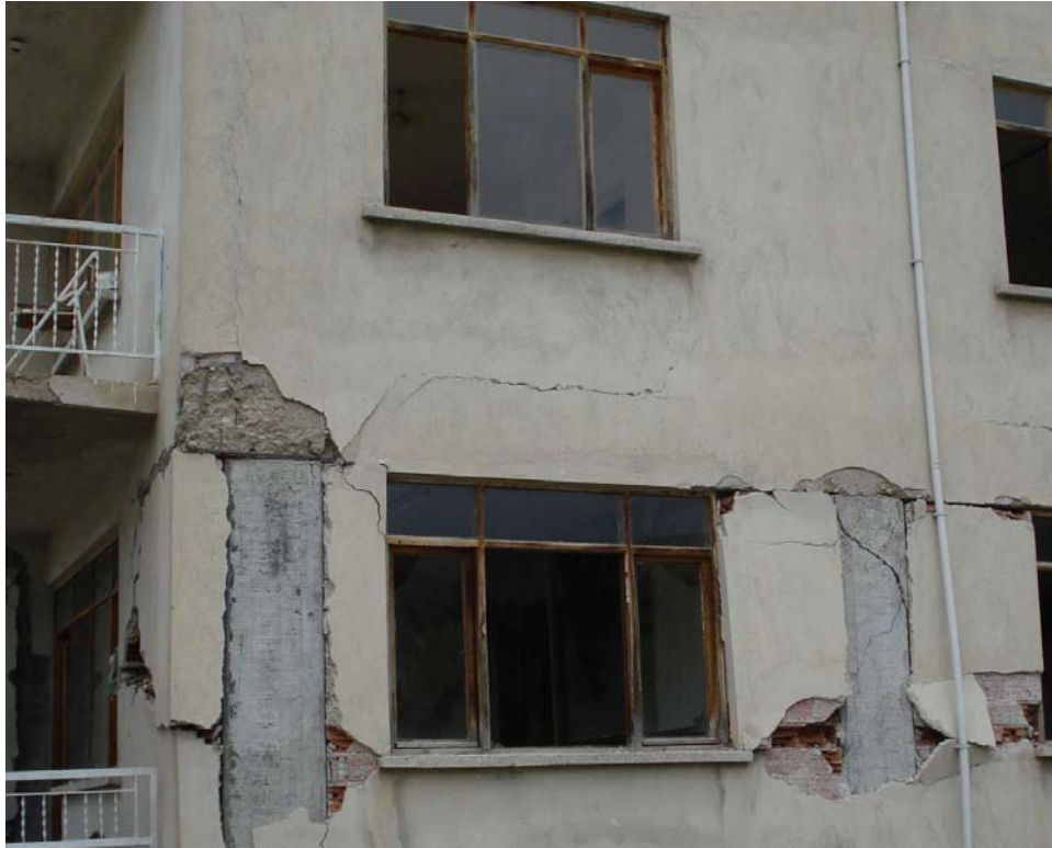
Figure 81: Gökçeler village, grade 3 damaged building, side view
