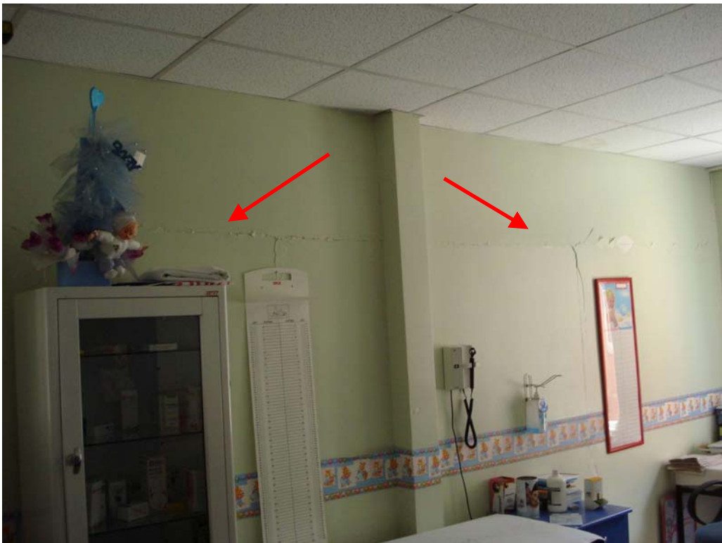
Figure 70: Hospital building, completed in the beginning of 2000's, infill wall crack
