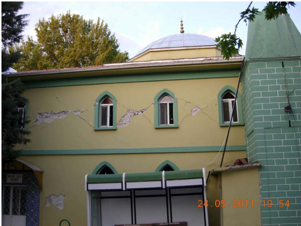
Figure 82: Cracks on brick masonry mosque
